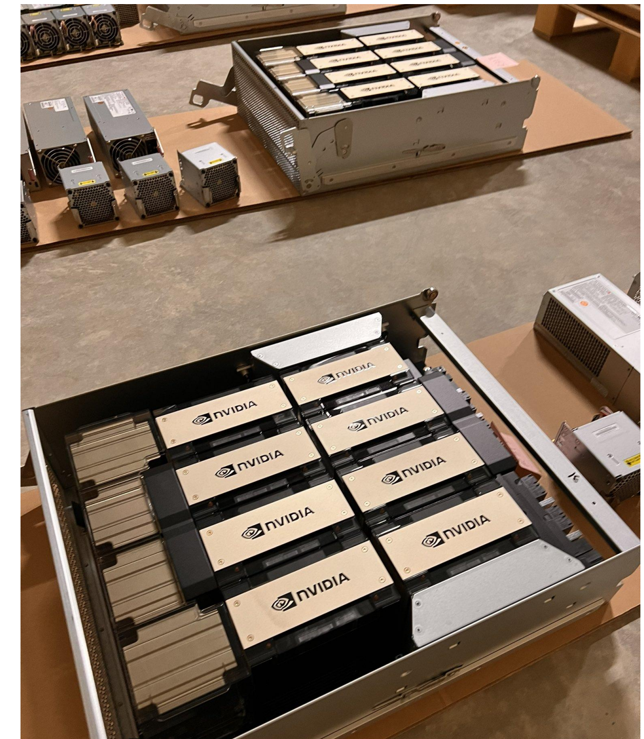
▲October 2023 Setting up GPU servers at Ishikari Data Center
